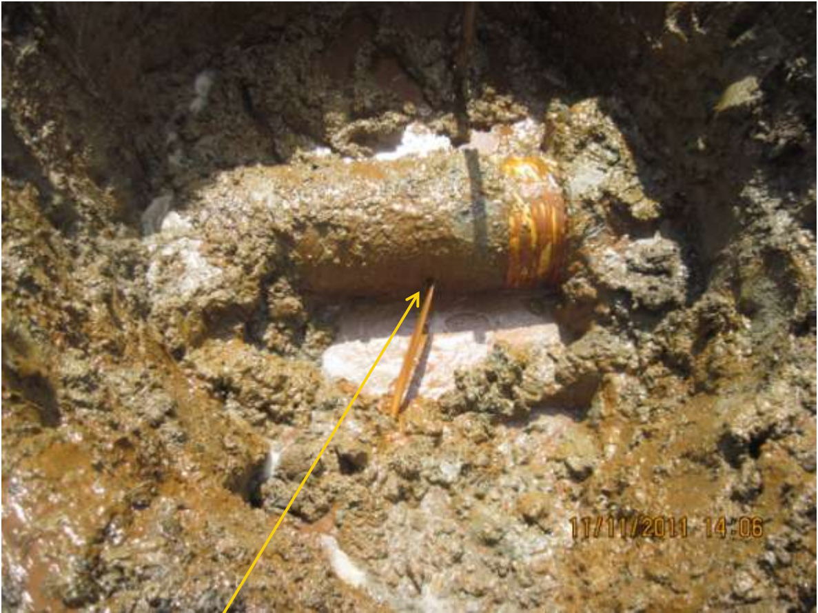
Close-up: Spill due to hacksaw cut on 14" Okordia-Rumuekpe pipeline at Ikarama. Picture was taken during Joint Investigation of 11 th November, 2011.
