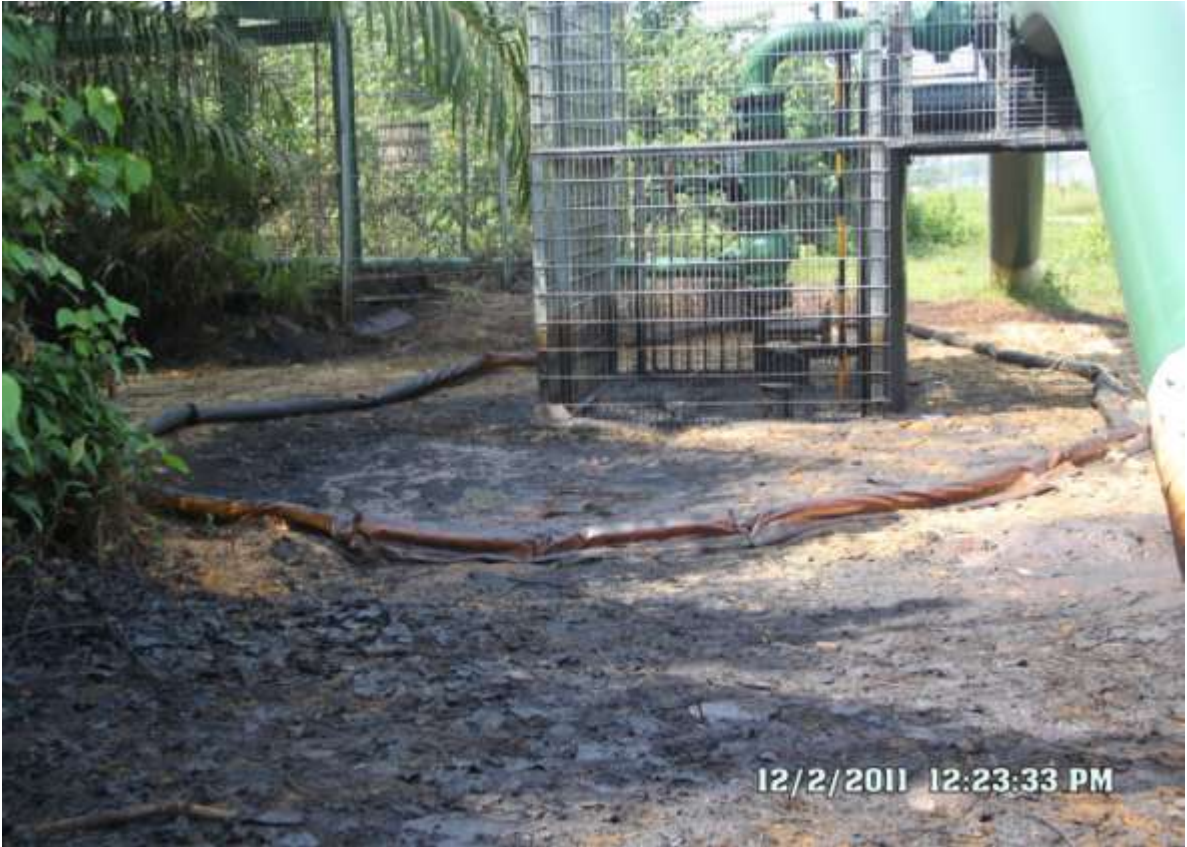
Overview: Part of spill impact on 8" North bank Tie-in Manifold. Picture was taken during Joint Investigation of 2 nd December, 2011.
