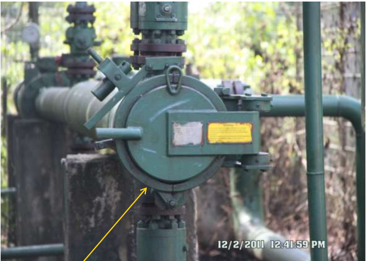
Close-up: Failed barrel door on 8" North bank Tie-in Manifold. Picture was taken during Joint Investigation of 2 nd December, 2011.
