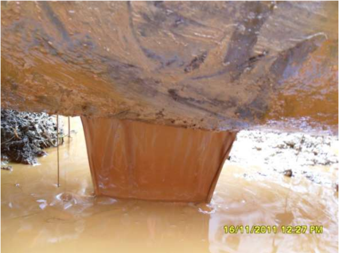
Close-up: Spill due to corrosion on 12" Adibawa-Okordia pipeline at Ikarama. Picture was taken during Joint Investigation of 16 th November, 2011.
