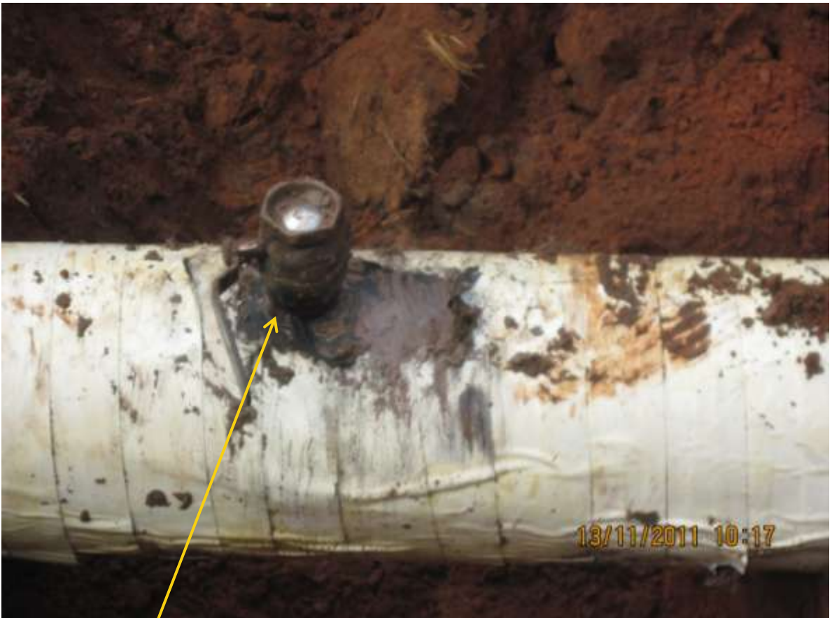
Close-up: Illegal fitting on 16" Egbema-Assa pipeline at Assa. Picture was taken during Joint Investigation of 13 th November, 2011.
