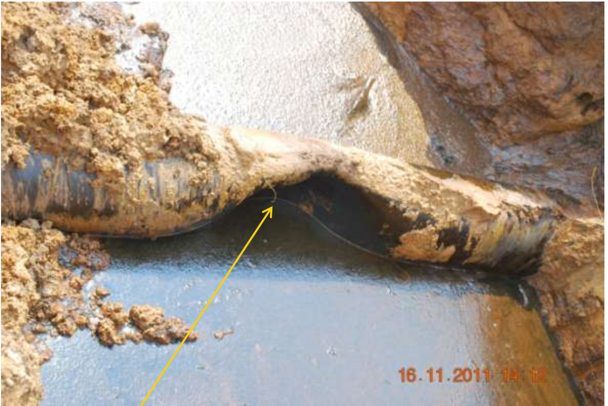
Close-up: Dent on 16" Uzere-Eriemu pipeline at Iyede. Picture was taken during Joint Investigation of 16 th November, 2011.
