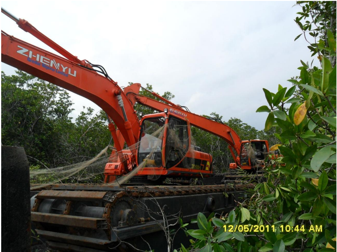
Overview: Swamp buggy at site covered with fishing nets placed by community members thus delaying response. Picture was taken during JIV of 12 th May, 2011
