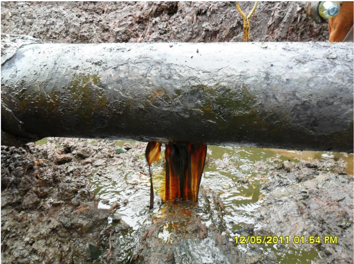
Close-up: Closeup of spill point on 10in Ekulama1 pipeline at Freetown. Picture was taken during JIV of 12 th May, 2011
