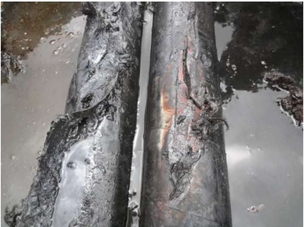
Close-up: Inward dent on the Cawthorne channel Well 29T flowline at Mbiama. Picture was taken during JIV of 18 May 2011
