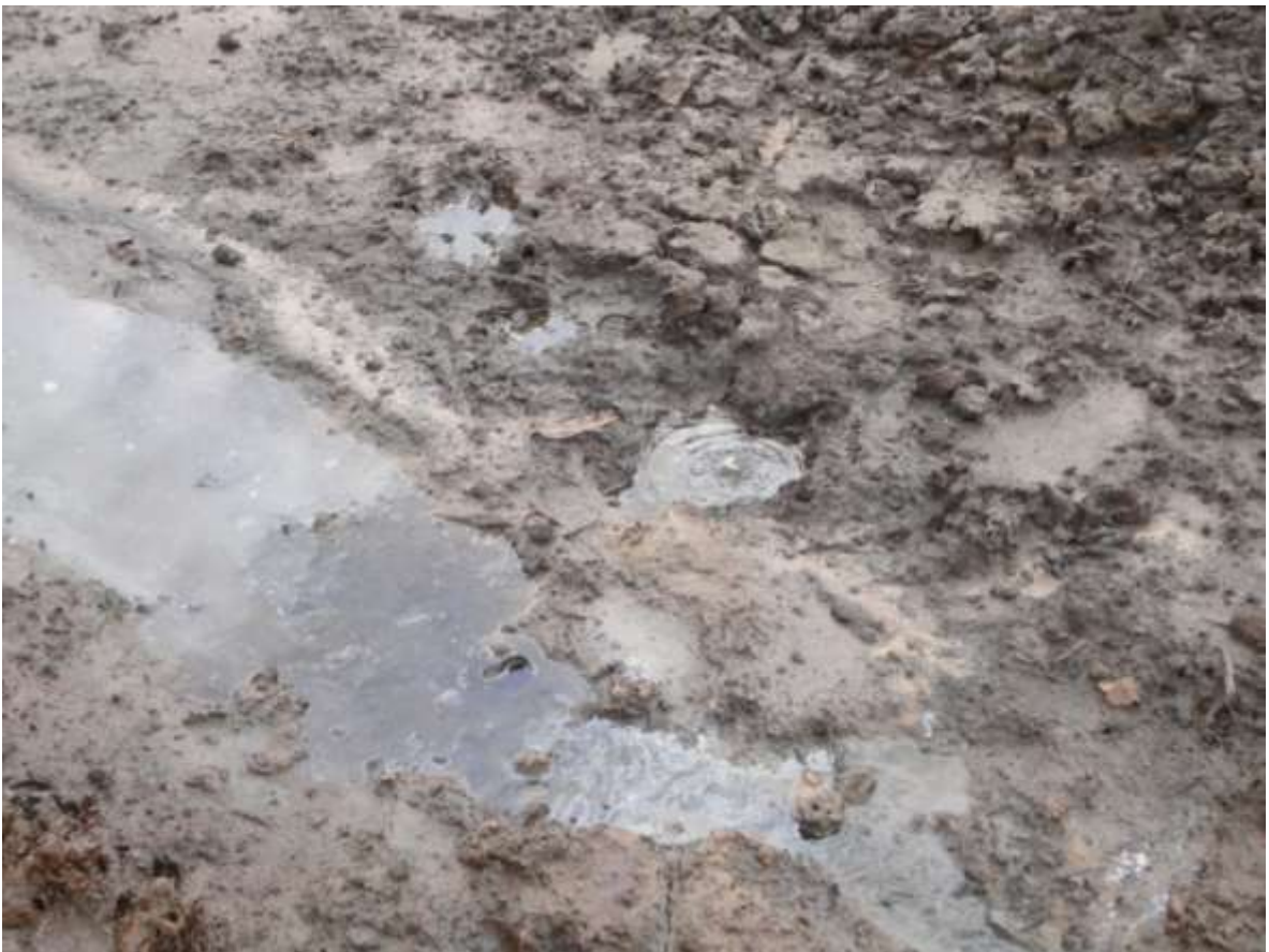
Overview: Spill point on the Cawthorne channel Well 29T flowline at Mbiama. Picture was taken during JIV of 18 May 2011
