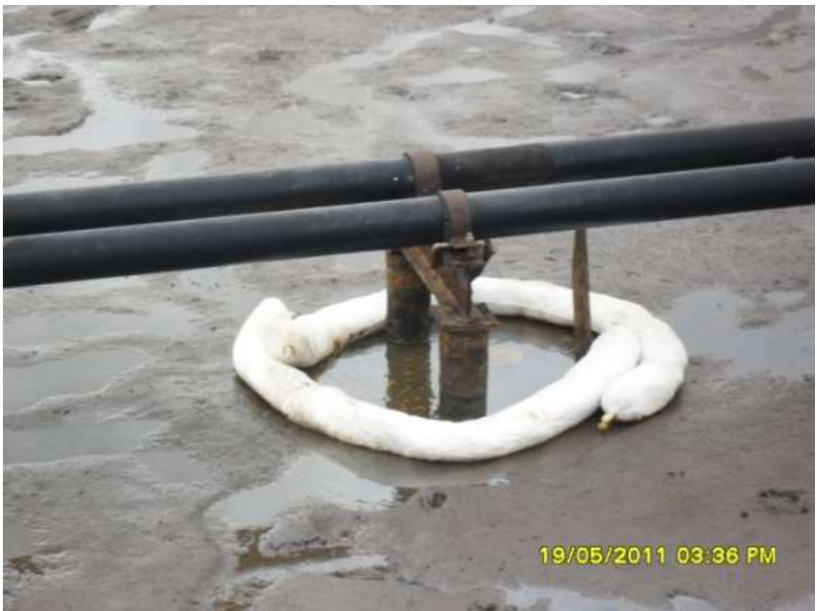
Overview: Extent of the spill incident impact at the 6" Awoba Pipeline route in Owaza . Picture was taken during JIV of 19 May 2011 .
