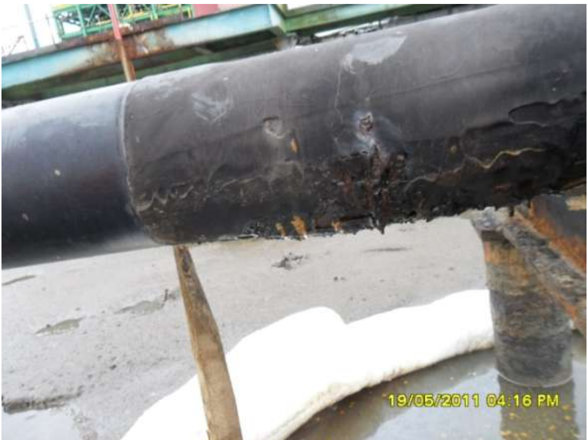
Close-up: Corrosion tear on the 6" Awoba Pipeline at Bille. Picture was taken during JIV of 19 May 2011 .
