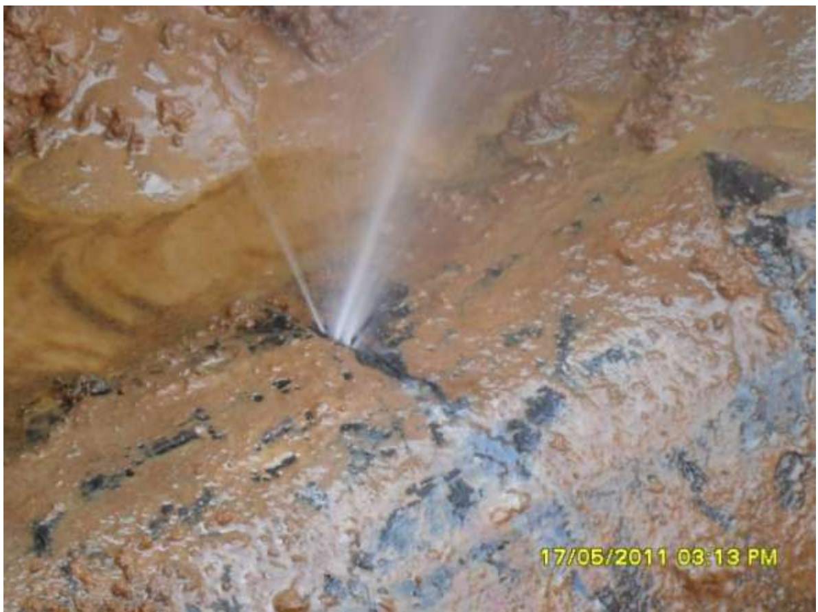
Close-up: Hacksaw cut on 18" Assa – Rumuekpe Pipeline at Egbeda. Picture was taken during JIV of 17 May 2011
