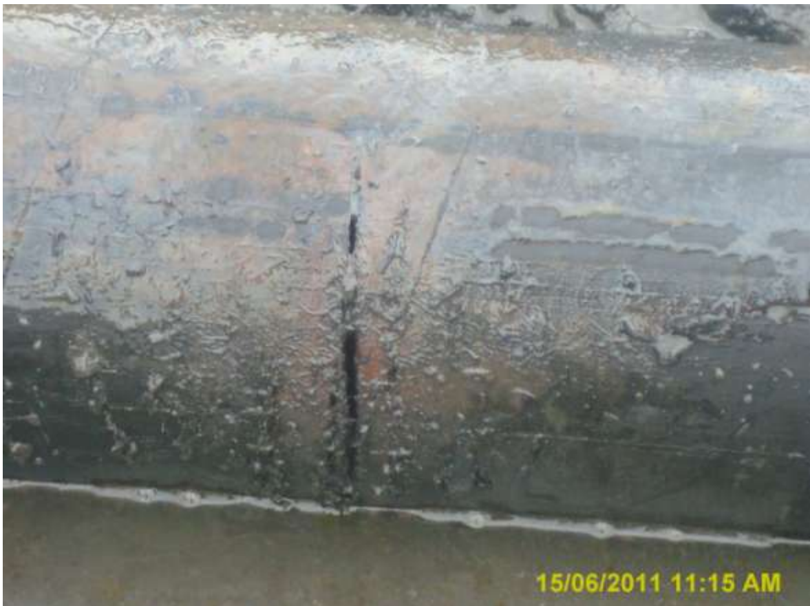
Close-up: Spill due to hacksaw cut on Bonny-Oloma Well 12S flowline at Oloma. Picture taken during Joint Investigation of 15 th June, 2011.
