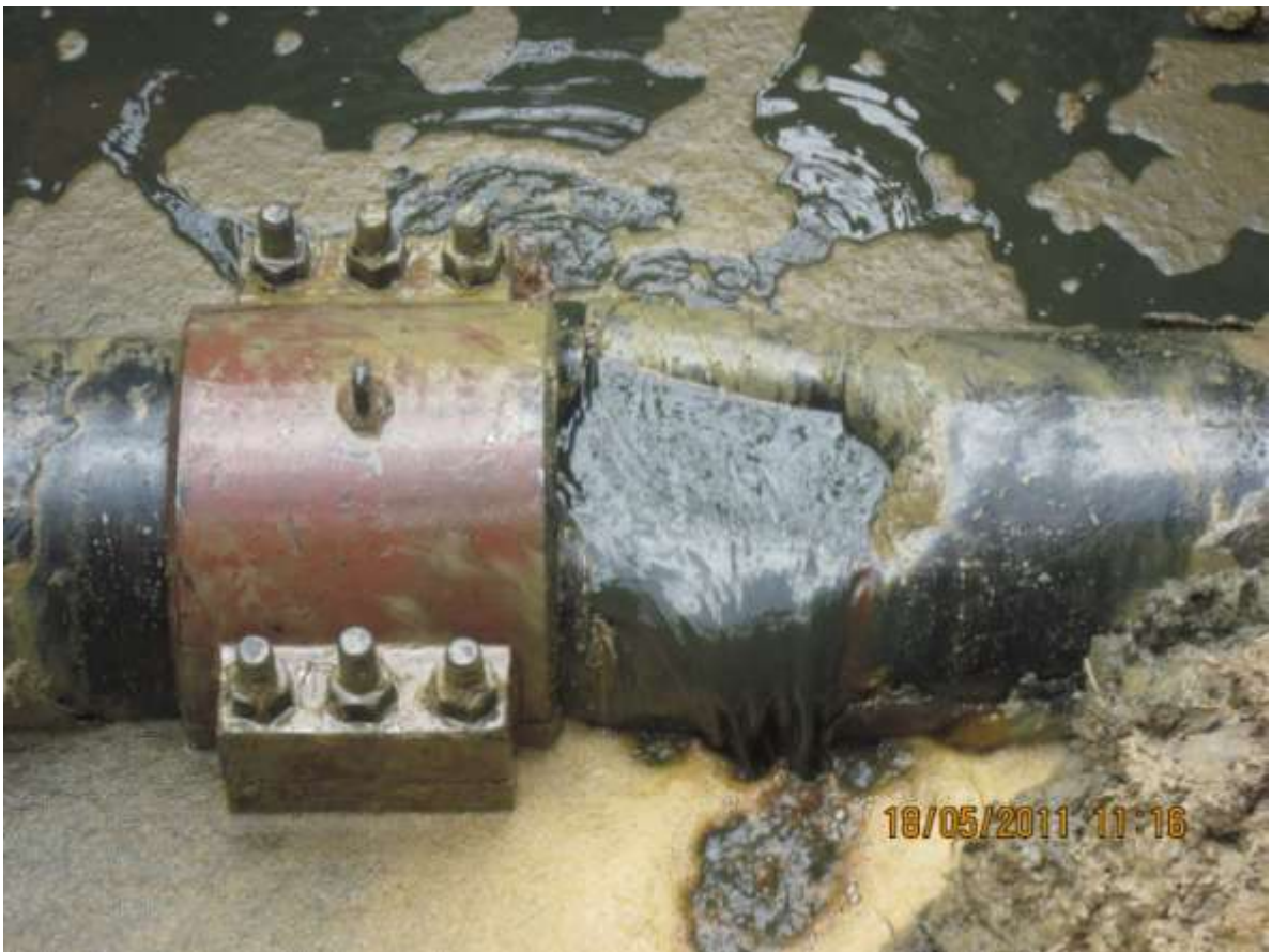
Close-up: Damage due to explosion evident on the 10 inch Diebu Creek – Nun river pipeline at Nun river. The visible clamp is from an earlier spill response.
