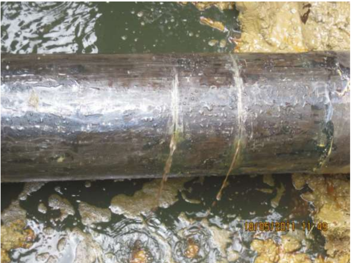
Close-up: Hacksaw cuts on the 10 inch Diebu Creek – Nun river pipeline at Nun river. Picture was taken during JIV of 18 May 2011.
