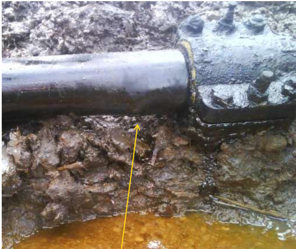
Close-up: Failed clamp point on Awoba NorthWest Well 1 L/S flow line at Boro. Picture was taken during JIV of 19 th May, 2011
