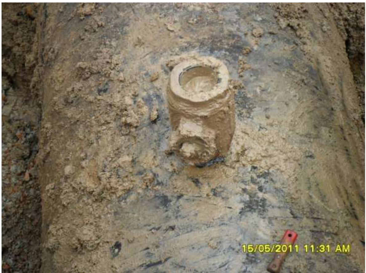
Close-up: Illegally welded point on Rumuekpe-Nkpoku pipeline at Rumuekpe. Picture was taken during JIV of 15 May 2011.
