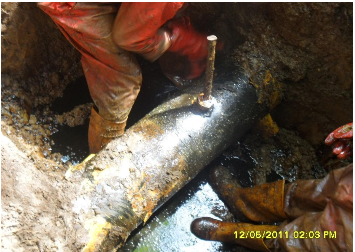
Overview: Illegally welded point on 12'' Imo River Pipeline at Owaza. Picture was taken during JIV of 12 th May, 2011
