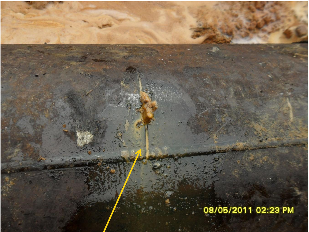
Close-up: Close up of hacksaw cut on 18in Assa-Rumekpe pipeline at Egbeda. Picture was taken during JIV of 8 th May, 2011.
