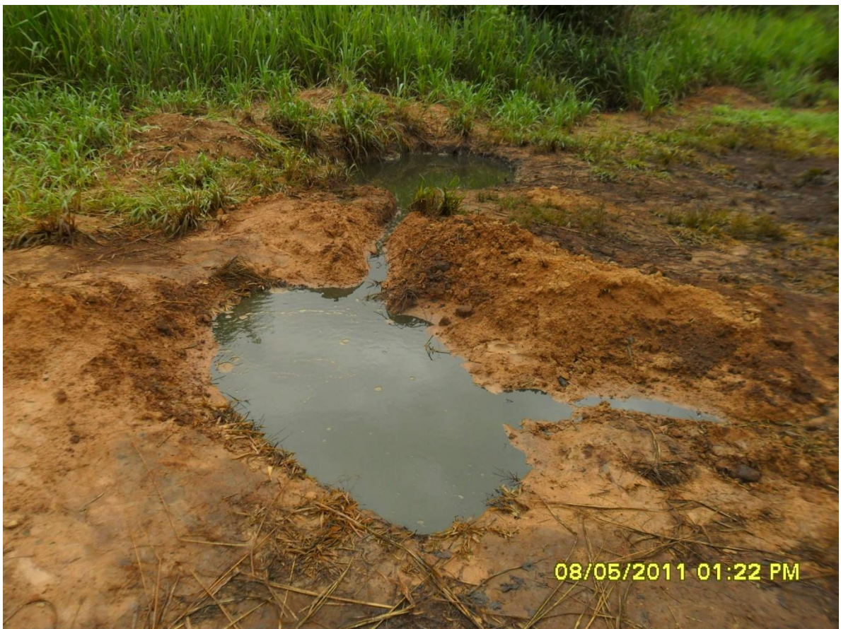
Overview: View of part of the spill incident on the 18in Assa-Rumekpe pipeline at Egbeda. Picture was taken during JIV of 8 th May, 2011
