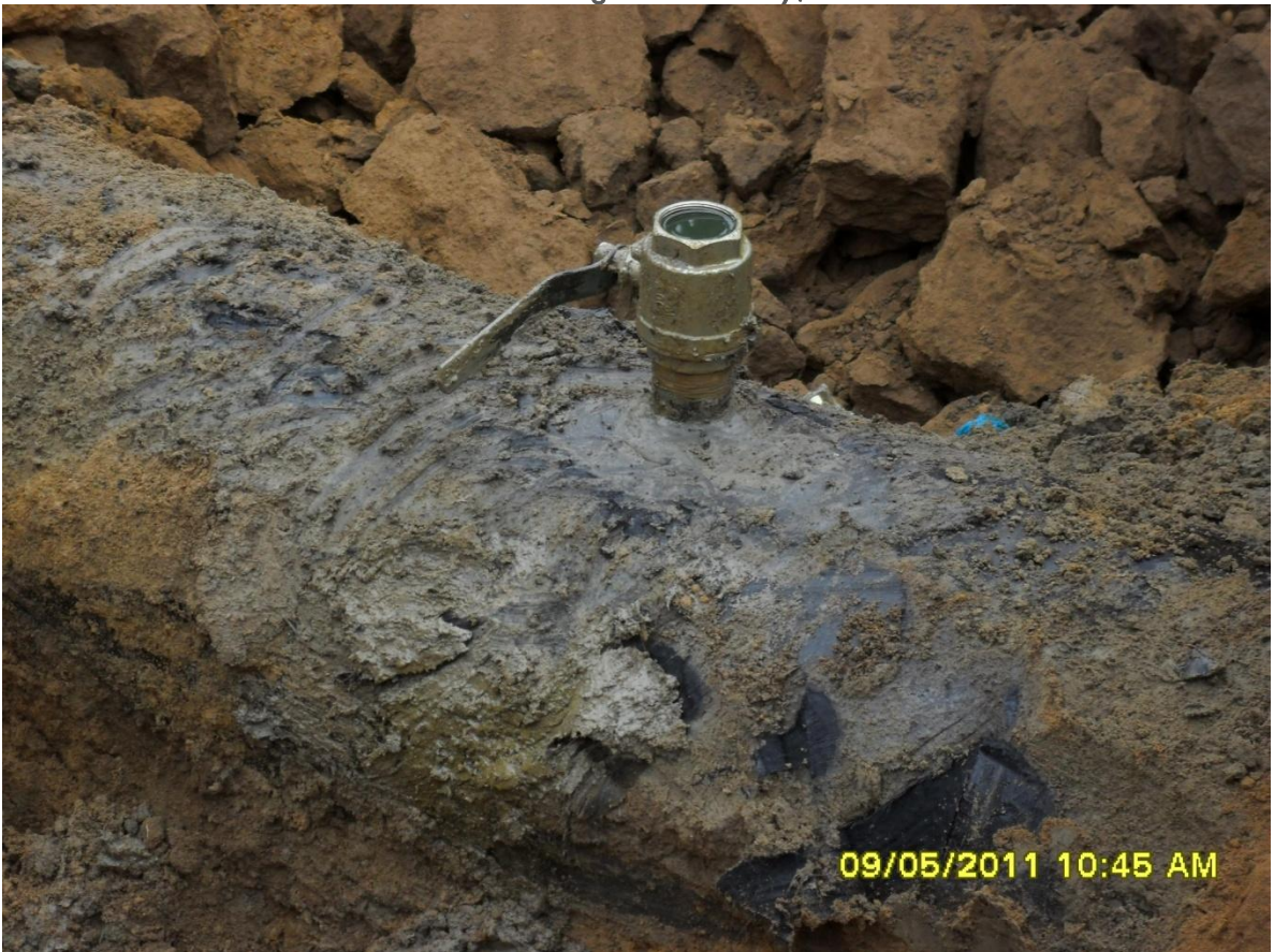
Close-up: Illegally welded point on on 18in Assa-Rumekpe pipeline at Egbeda. Picture was taken during JIV of 9 th May, 2011.
