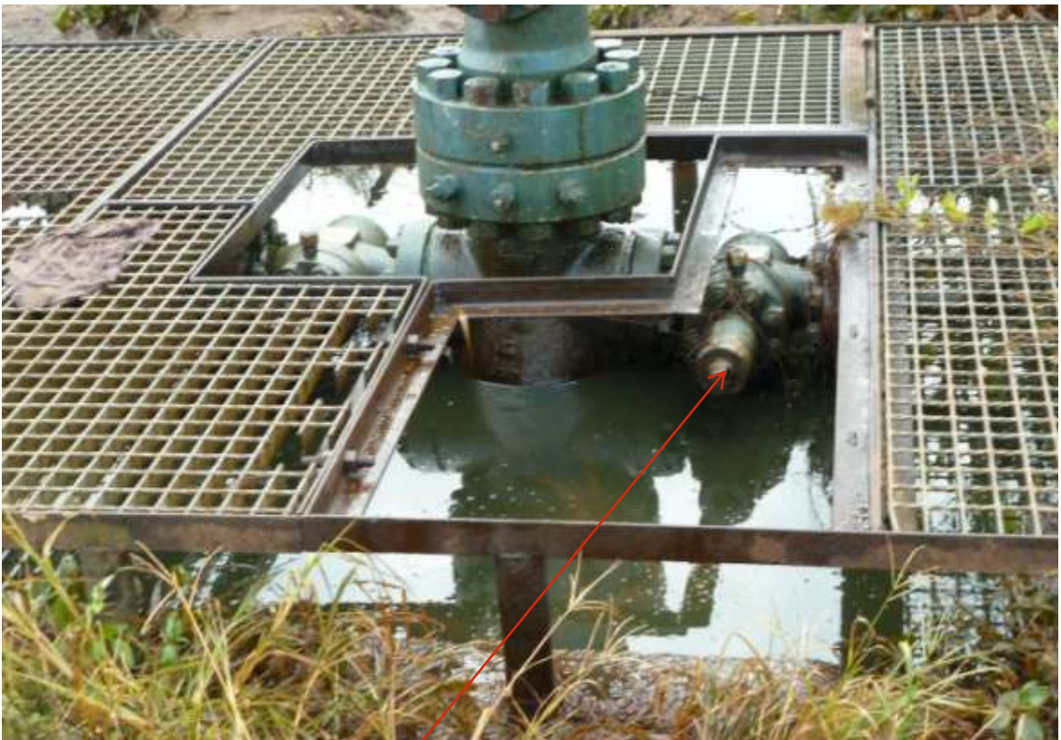
Close-up: Tampering with well Head Valve setting on Apra Well 3L Well Head in Rumuola/Rumudaolu. Picture was taken during JIV of 10 th May, 2011
