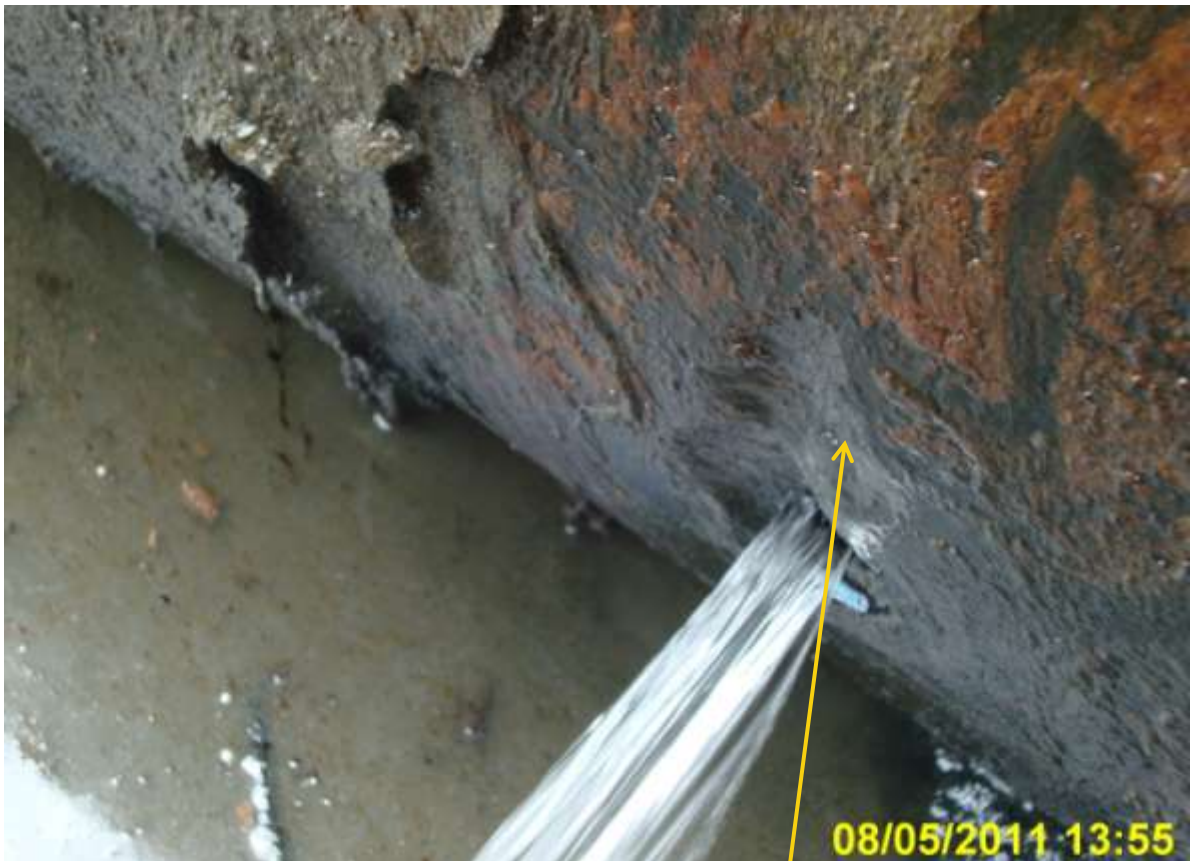
Close-up: Evidence of grinding and drilled hole on 24" Alakiri-Bonny Pipeline at Kalibiama. Picture was taken during JIV of 8 th May 2011
