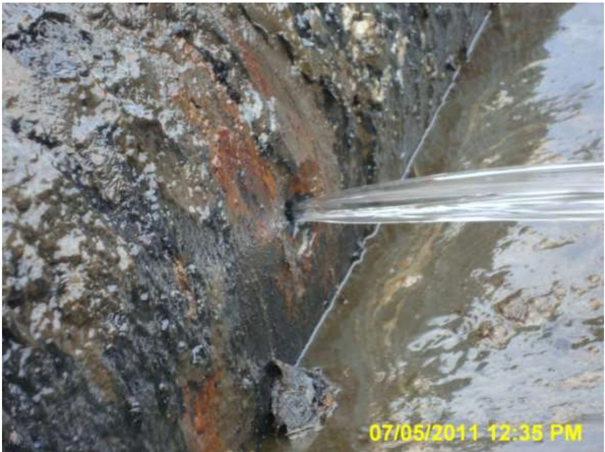
Close-up: Evidence of mechanical grinding on the surface of the 24" Alakiri-Bonny Pipeline in Creek 6. Picture was taken during JIV of 7 th May 2011
