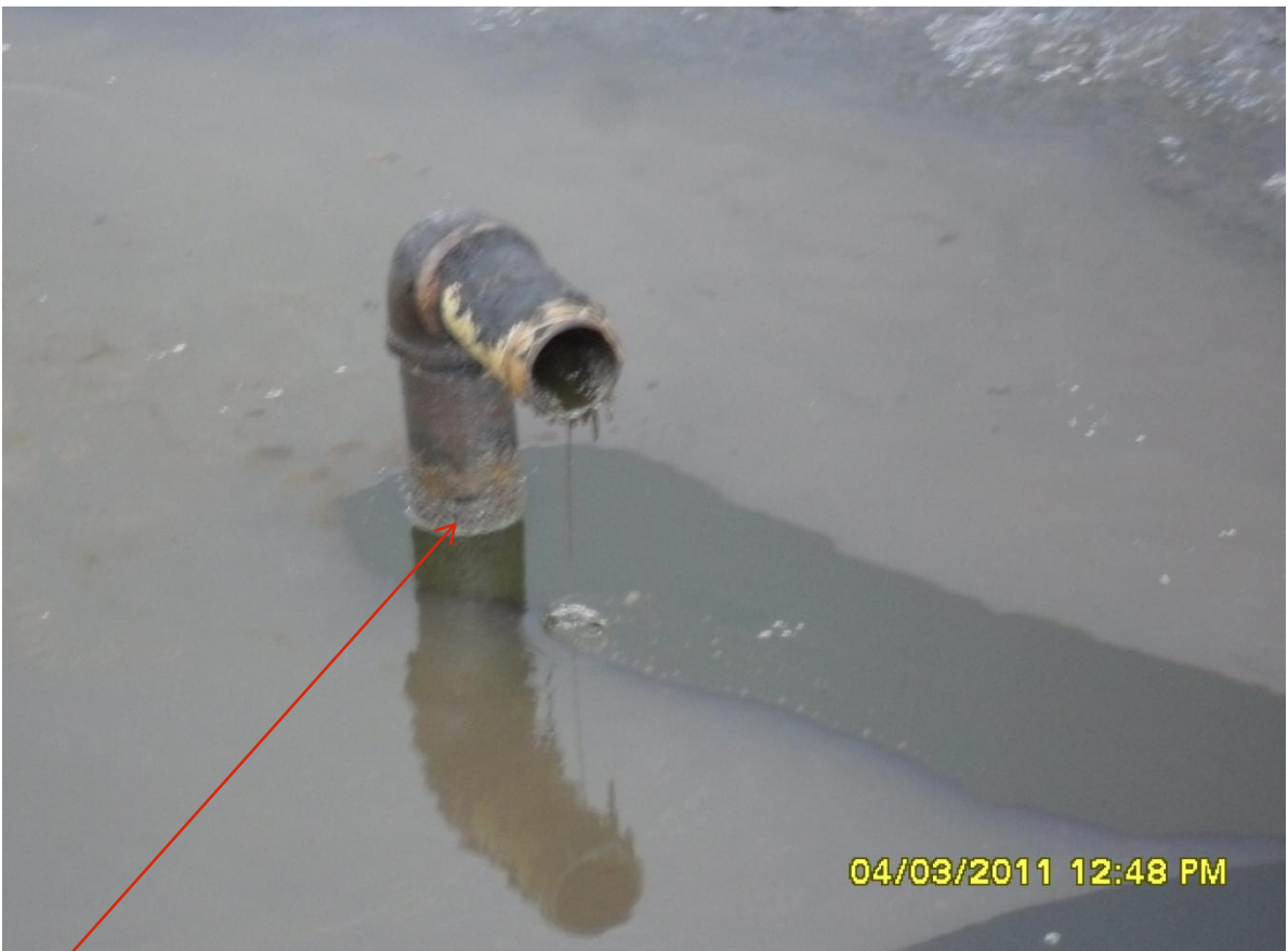
Close-up: Spill due to illegally welded points on 18" Soku - Ekulama Pipeline at Kirikakiri. Picture taken during Joint Investigation of 4 th March, 2011.
