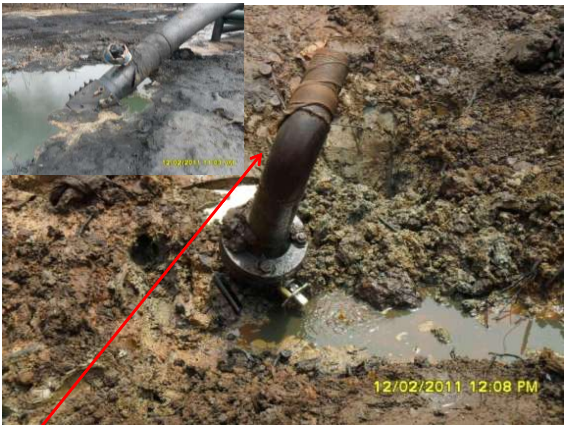
Close-up: Illegally welded points on 20" Kolocreek – Rumuekpe Pipeline in Ogbogolo. Picture was taken during JIV of 12 February 2011
