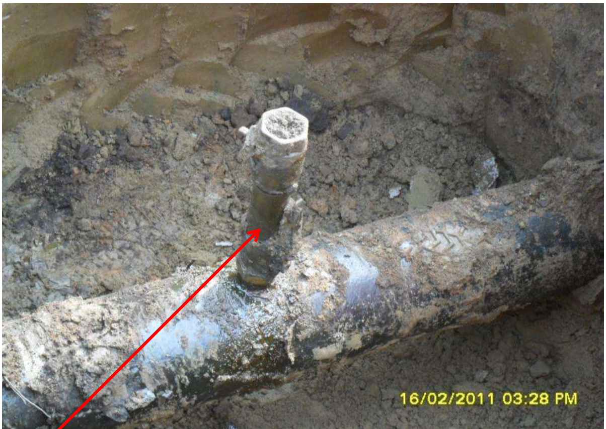
Close-up: Illegally welded point on 8" Obigbo-North Pipeline in Obigbo. Picture was taken during JIV of 16 February 2011
