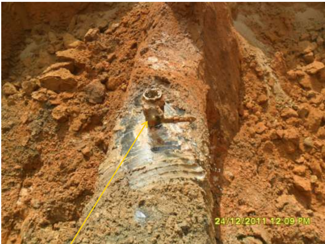
Close-up: Illegal fitting on 18" Assa-Rumuekpe pipeline at Awara. Picture was taken during Joint Investigation of 24 th December 2011.
