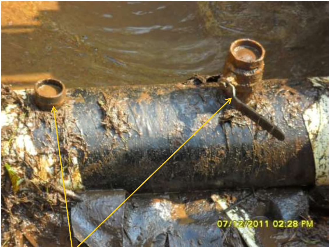
Close-up: Illegal fittings on 12" Imo River1 – Ogale pipeline at KomKom. Picture was taken during Joint Investigation of 7 th December, 2011.
