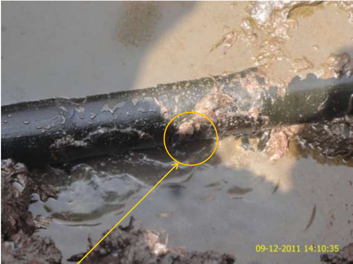
Close-up: General location of tear at 6'o clock position on Bonny-Oloma Well2L flowline at Oloma. Picture was taken during Joint Investigation of 9 th December, 2011.
