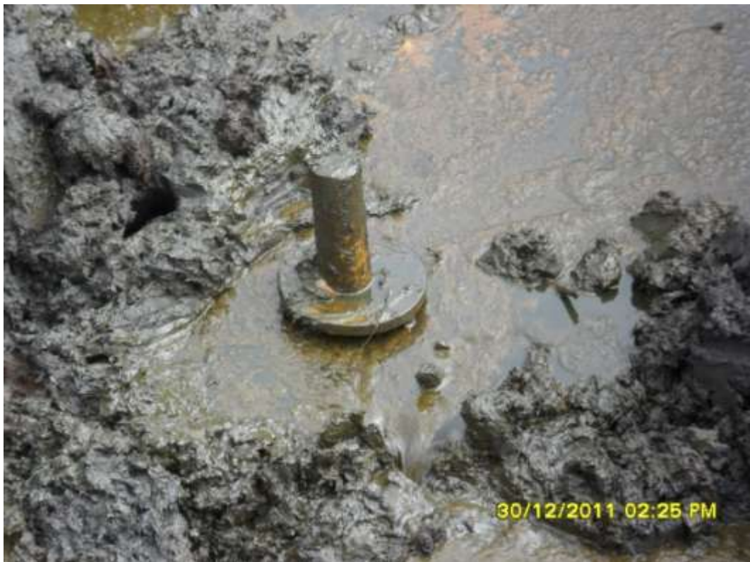
Close-up: Illegal fitting on 24" Nembe Creek pipeline at Nembe Bassambiri. Picture was taken during Joint Investigation of 30 th December 2011.
