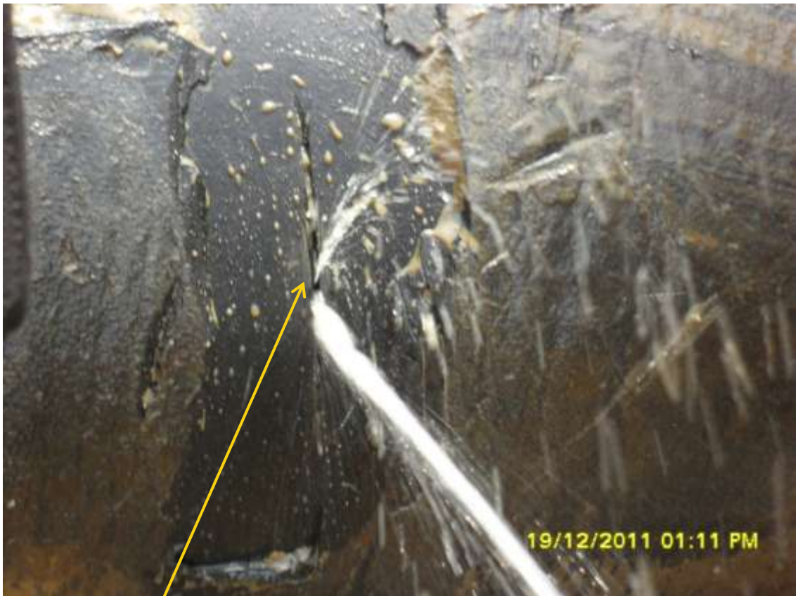
Close-up: Hacksaw cut on 16" NunRiver-Kolocreek pipeline at Aguobiri. Picture was taken during Joint Investigation of 19 th December, 2011.
