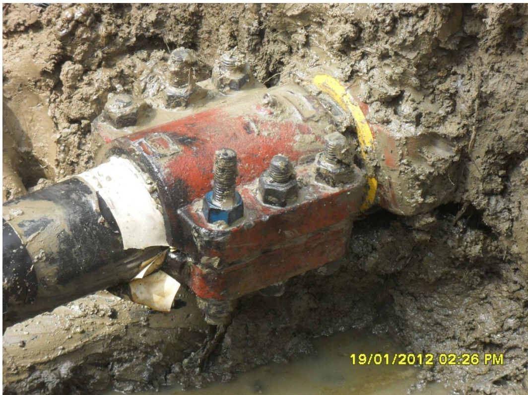
Close-up: Spill due to failed damp on Nun River Well 15S flowline at Onyoma. Picture was taken during Joint Investigation of 19 th January 2012.
