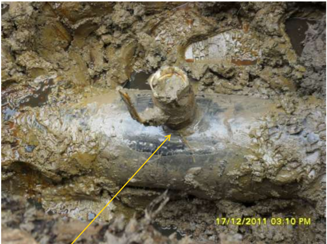
Close-up: Spill due to illegal fitting on 10" Diebu Creek pipeline at Oporoma. Picture was taken during Joint Investigation of 17 th December, 2011.
