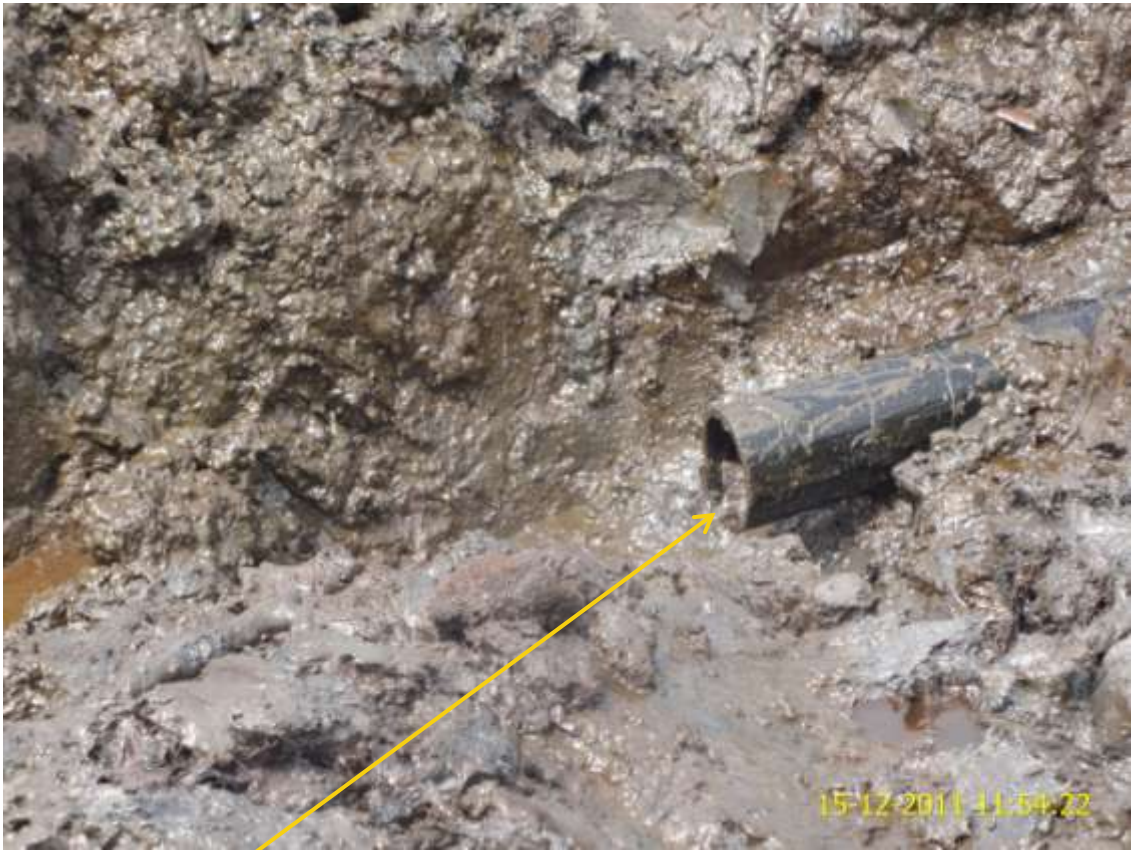
Close-up: Cut section on Akaso Well3S flowline at Ilomatoru. Picture was taken during Joint Investigation of 15 th December, 2011.
