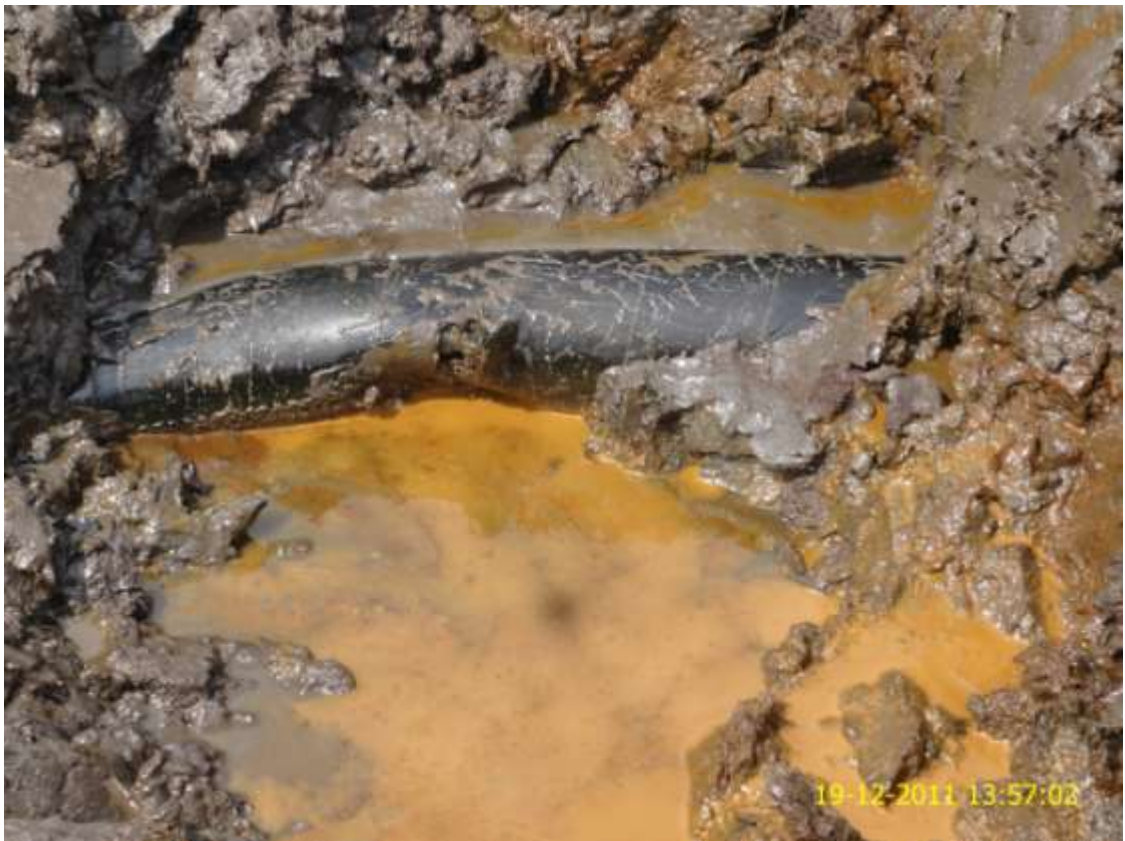
Close-up: Outward dent on Ekulama1 Well35S flowline at SandSand. Picture was taken during Joint Investigation of 19 th December 2011.
