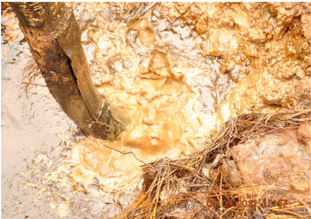
Close-up: Spill due to Complete Rupture on Ogini Well 4T 4" Flowline at Ovrode. Picture taken during Joint Investigation of 9 th September, 2011
