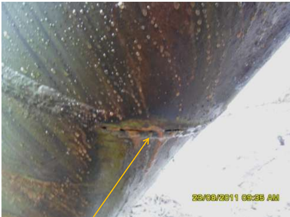
Close-up: Spill due to hacksaw cut on Buguma-Alakiri trunkline right of way at Abiama. Picture taken during Joint Investigation of 23 rd August, 2011.
