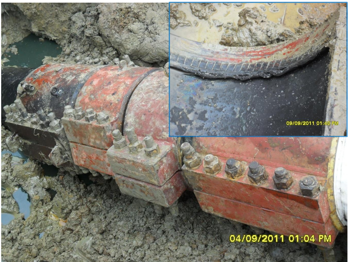
Close-up: Spill due to failed clamp point on 20" Kolocreek – Rumuekpe Pipeline at Ogbogolo. Insert shows broken seal of failed clamp. Pictures were taken during JIV of 4th and 9 – 11th September, 2011.
