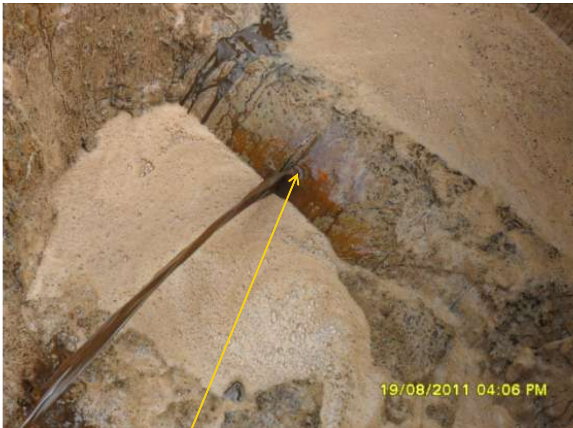
Close-up: Spill due to hacksaw cut on 14in Okordia-Rumuekpe pipeline at Ikarama. Picture taken during Joint Investigation of 19 th August, 2011.
