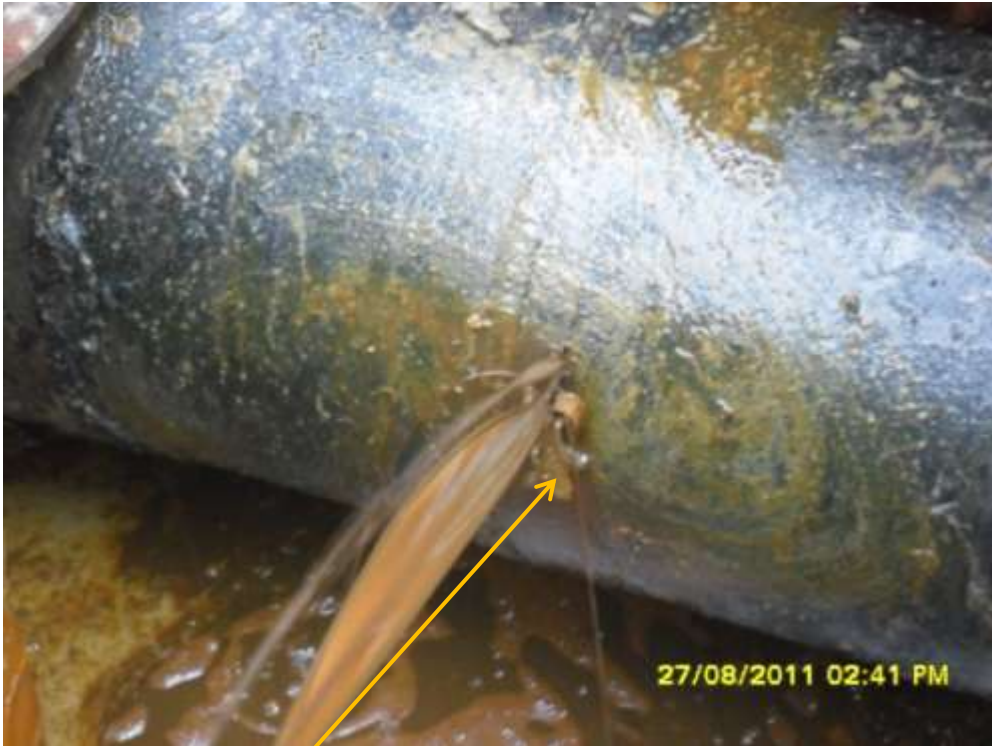
Close-up: Spill due to hacksaw cut on 12" Adibawa-Okordia pipeline at Ikarama. Picture taken during Joint Investigation of 27 th August, 2011.
