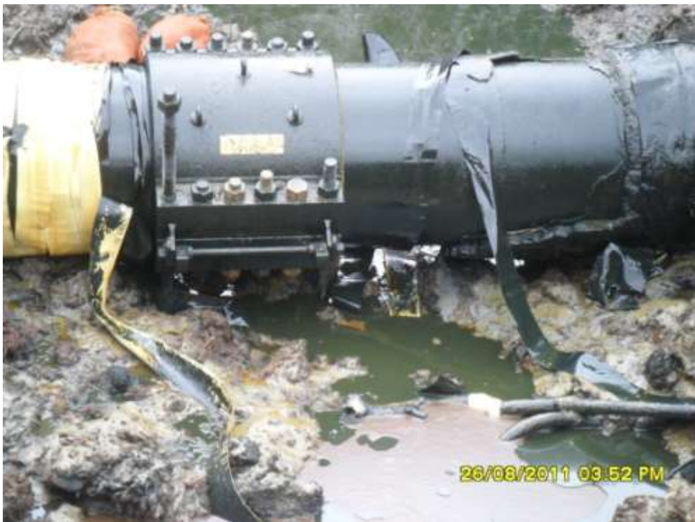
Close-up: Spill due to clamp failure on 24" Nembe Creek pipeline at Tora-Twenikiri. Picture taken during Joint Investigation of 26 th August, 2011.
