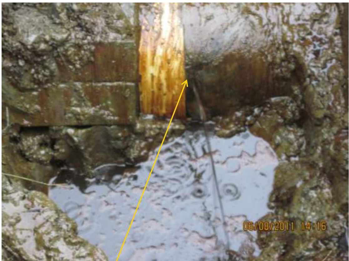
Close-up: Spill due to hacksaw cut on 14in Okordia-Rumuekpe pipeline at Ikarama. Picture taken during Joint Investigation of 6 th August, 2011.
