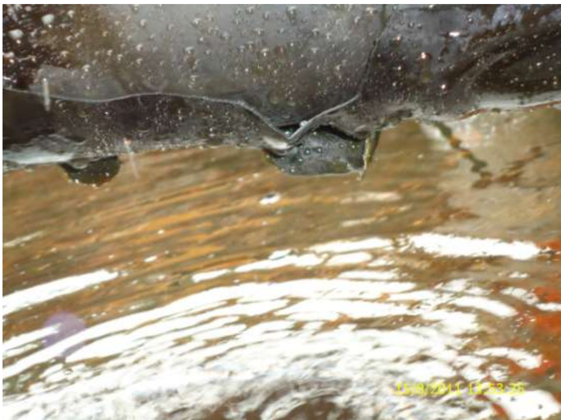
Close-up: Spill due to corrosion on Yokri Well 114S flowline at Yokri/Sokebolou. Picture taken during Joint Investigation of 15 th August, 2011
