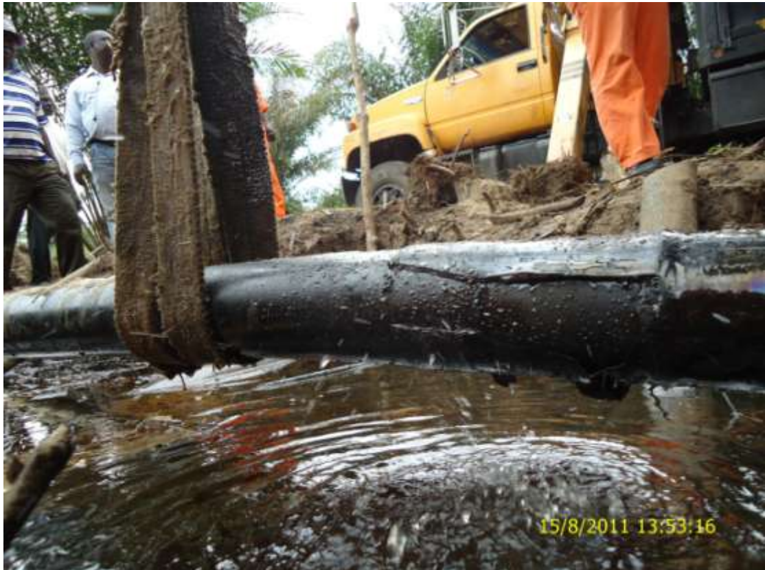
Overview: Yokri Well 114S flowline at Yokri/Sokebolou being raised for inspection. Picture taken during Joint Investigation of 15 th August, 2011
