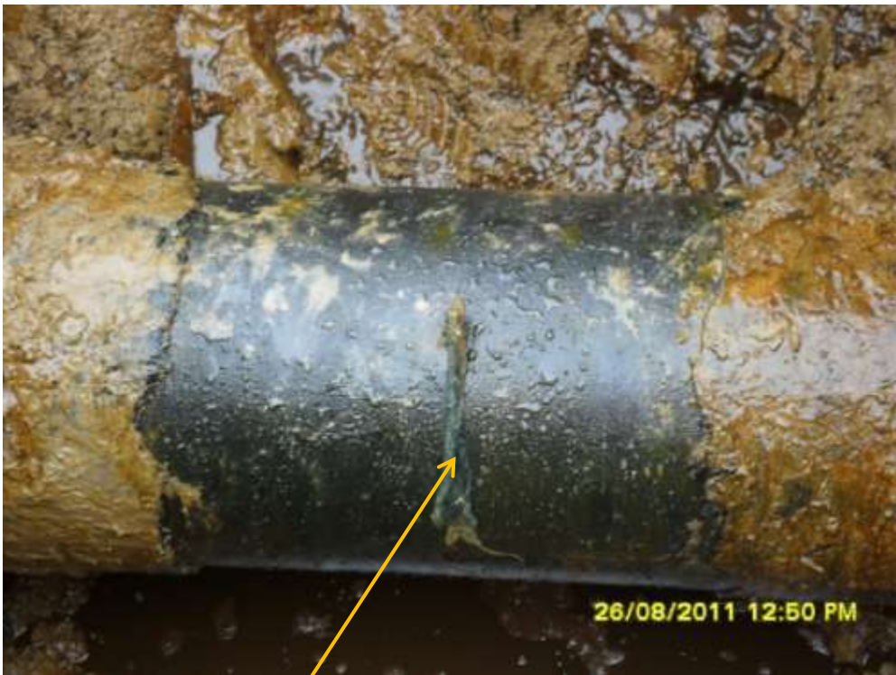
Close-up: Spill due to hacksaw cut on 12" Adibawa-Okordia pipeline at Ikarama. Picture taken during Joint Investigation of 26 th August, 2011.
