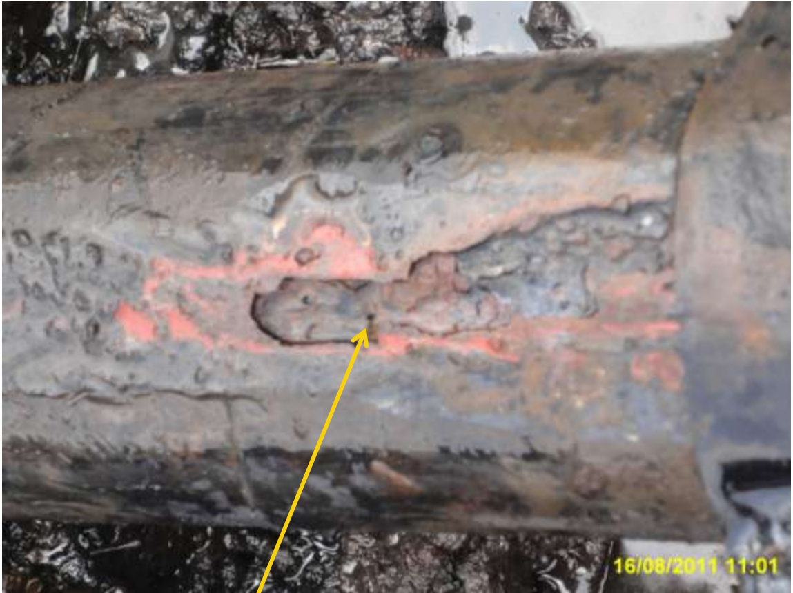
Close-up: Spill due to pinhole from inward dent on Cawthorne Channel Well 29T flowline at Mbiama. Picture taken during Joint Investigation of 16 th August, 2011.
