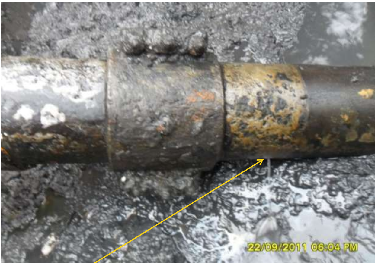
Close-up: Spill point due to corrosion on 10" Ekulama-Sanbarth pipeline at Sanbarth. Picture taken during Joint Investigation of 22 nd September, 2011
