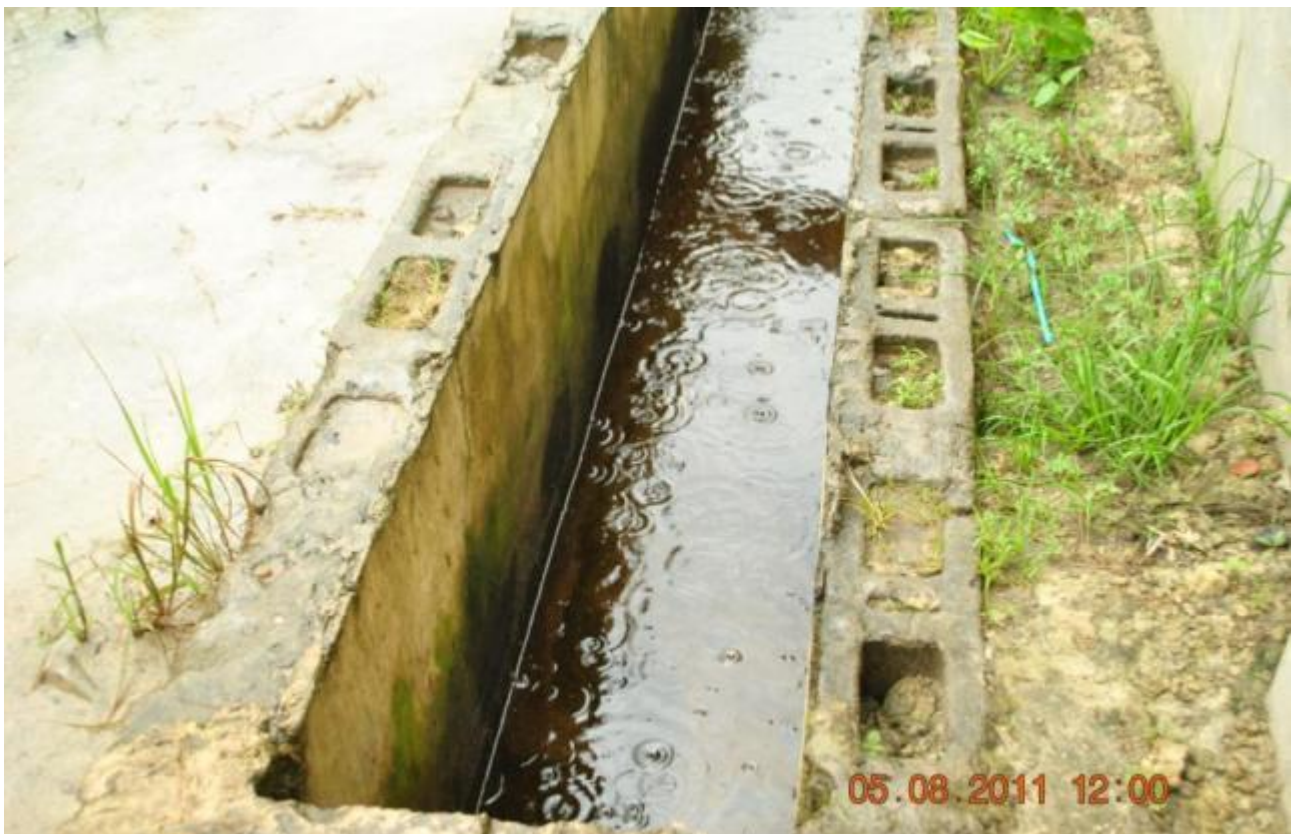
Overview: Part of spill impact on Ughelli Pumping Station-Warri Refinery Pipeline at Ekpan. Picture taken during Joint Investigation of 5 th August, 2011
