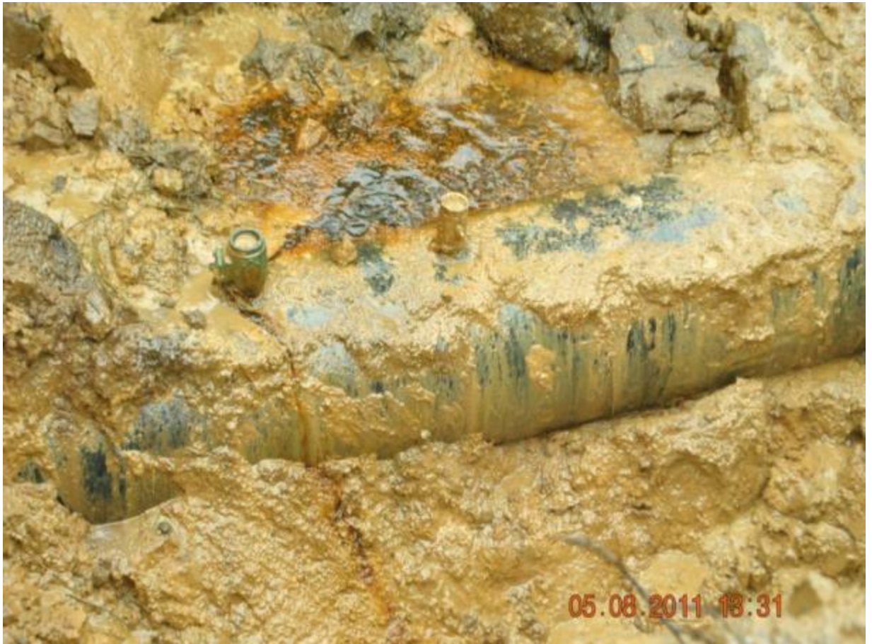
Close-up: Spill point on Ughelli Pumping Station-Warri Refinery Pipeline at Ekpan. Picture taken during Joint Investigation of 5 th August, 2011
