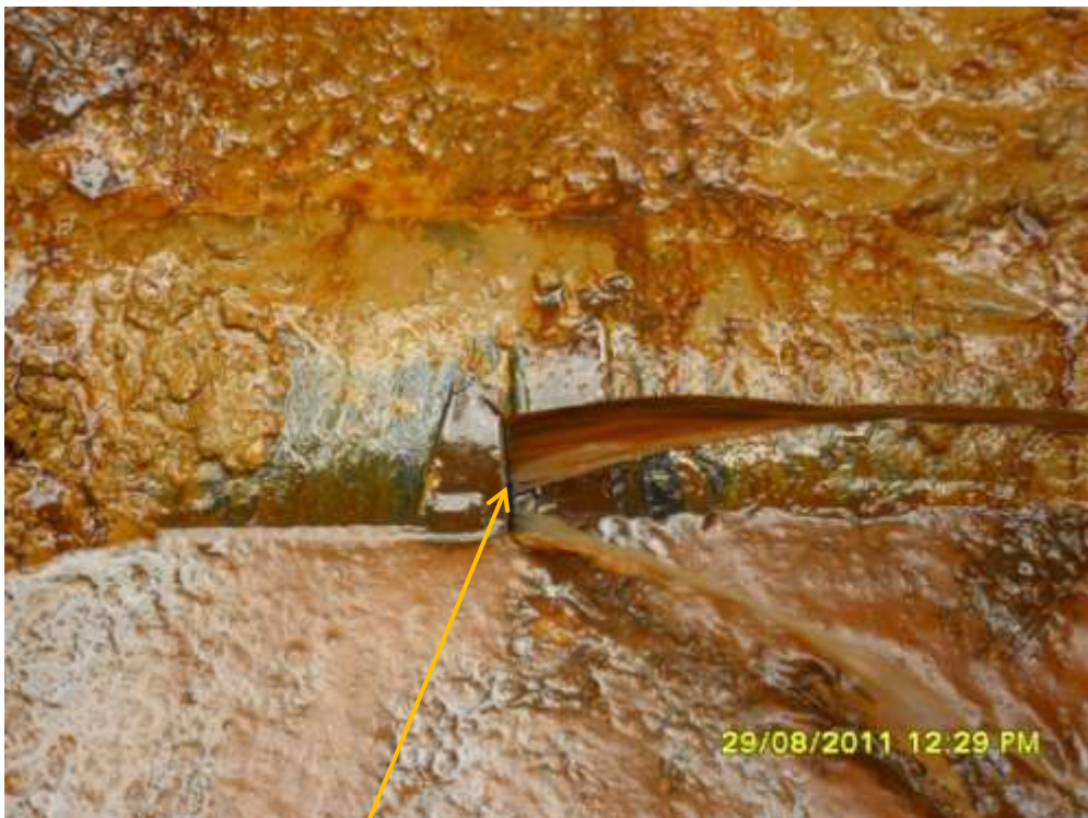
Close-up: Spill due to hacksaw cut on 14" Okordia-Rumuekpe pipeline at Ikarama. Picture taken during Joint Investigation of 29 th August, 2011.
