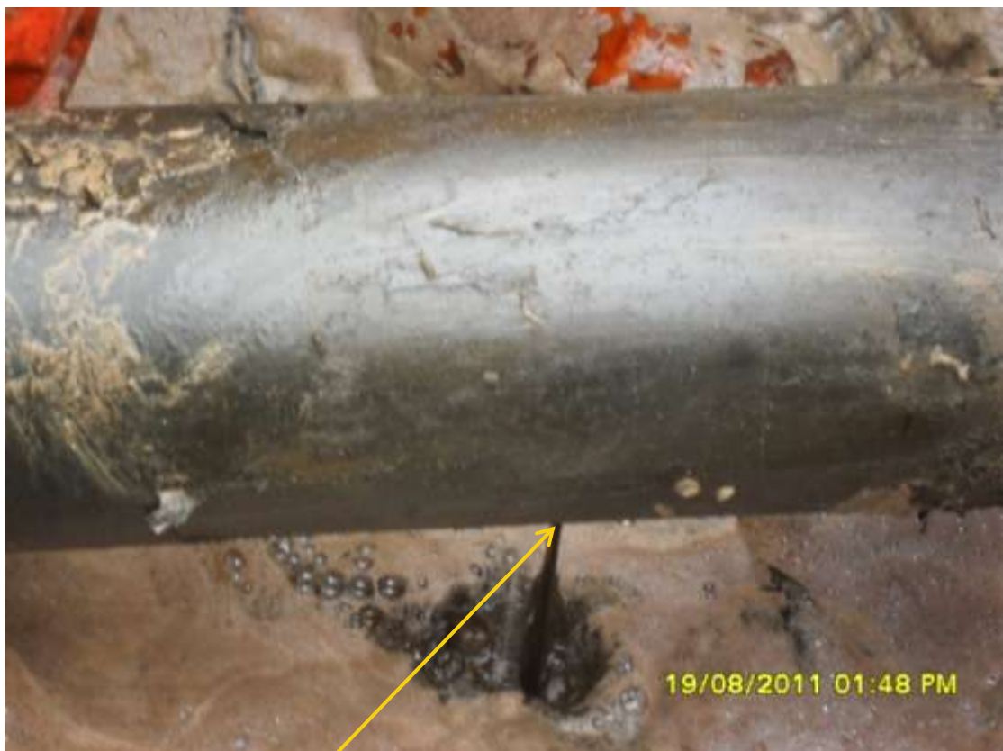
Close-up: Spill due to corrosion on 8" Obigbo North New Elenwo pipeline at Akpajo. Picture taken during Joint Investigation of 19 th August, 2011.
