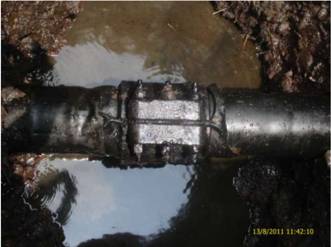
Close-up: Spill due to failed clamp on Cawthorne Channel Well 45T flowline at Mbiama. Picture taken during Joint Investigation of 13 th August, 2011.
