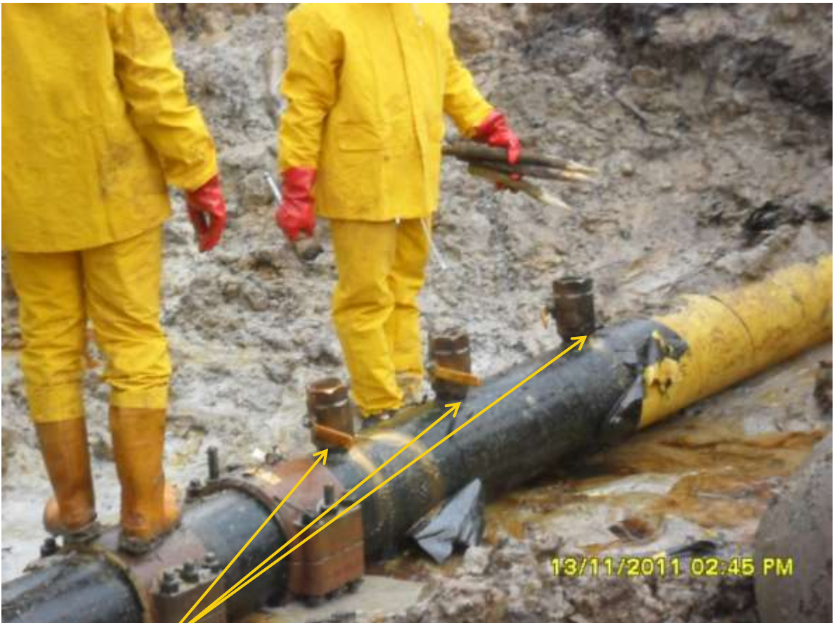
Close-up: Illegal fittings on 12" ImoRiver-Ogale pipeline at KomKom. Picture was taken during Joint Investigation of 13 th November, 2011.
