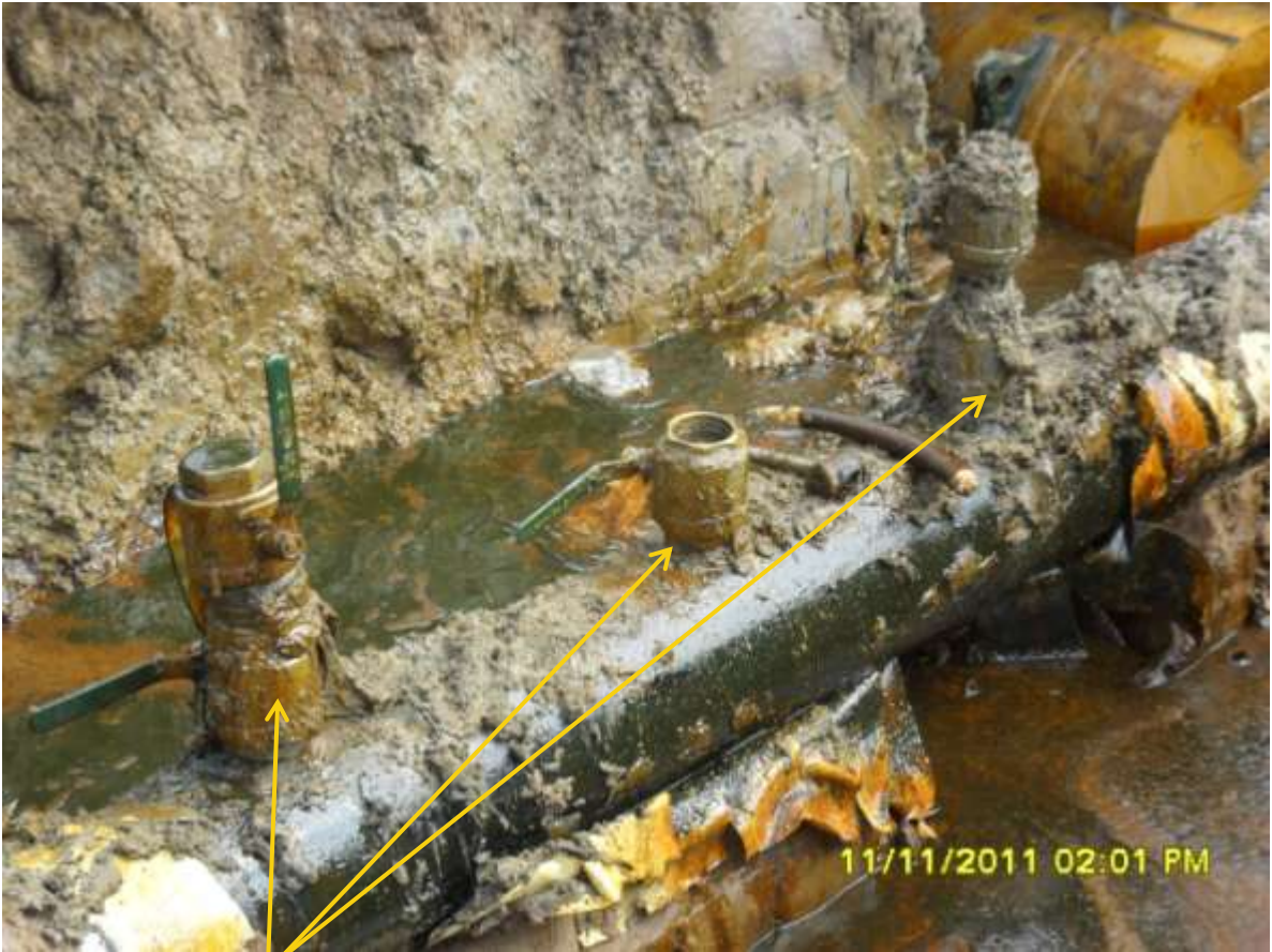
Close-up: Illegal fittings on 12" ImoRiver-Ogale pipeline at KomKom. Picture was taken during Joint Investigation of 11 th November, 2011.
