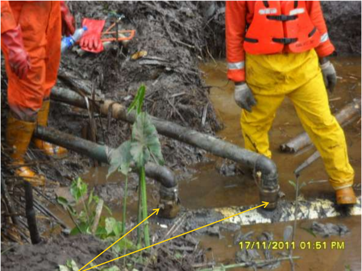
Close-up: Illegal fittings on 12" ImoRiver-Ogale pipeline at KomKom. Picture was taken during Joint Investigation of 17 th November, 2011.
