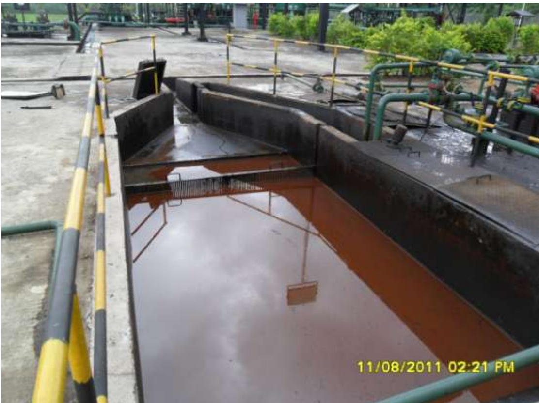
Close-up: Spill due to sump pit overflow at Obelle Flowstation at Obelle. Picture taken during Joint Investigation of 11 th August 2011.
