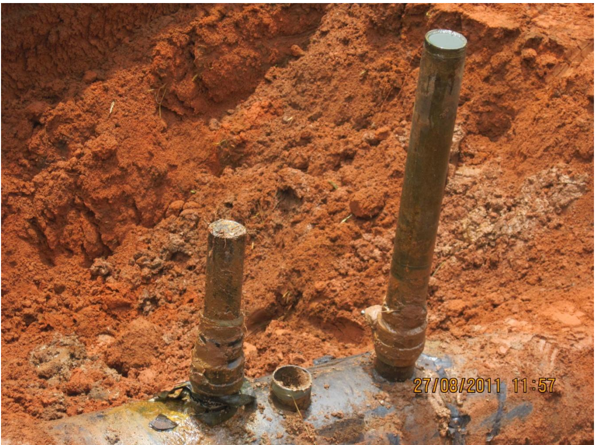
Close-up: Spill due to illegal fitting on 16'' Egbema -Asa Pipeline at Ekpeagha . Picture taken during Joint Investigation of 27-28 th August, 2011
