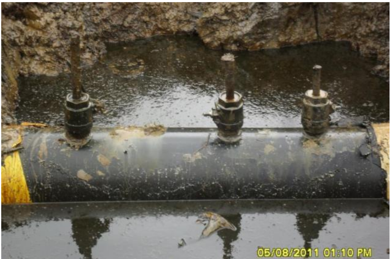
Close-up: Illegally welded points on 12" Imo River-Ogale Pipeline at Komkom . Picture taken during Joint Investigation on 5 th August, 2011
