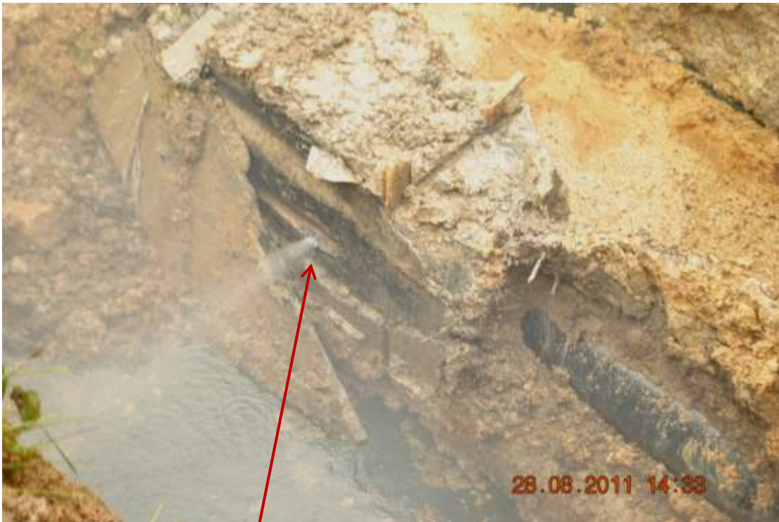
Close-up: Spill due to clamp failure on 10" Utorogu-UPS at Ughevwighe. Picture taken during Joint Investigation of 28 th August, 2011.
