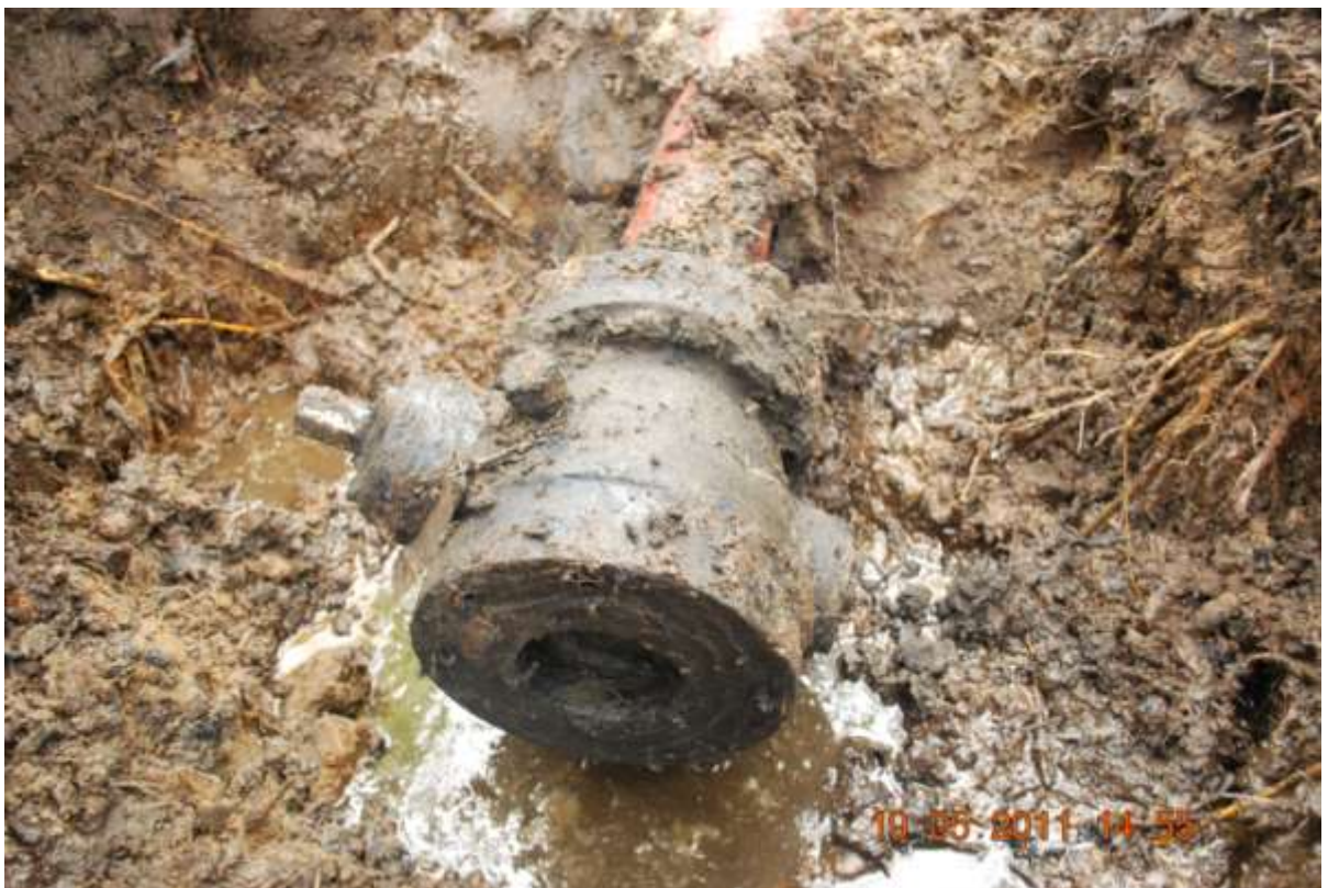
Close up: Illegal outlet flange on 24" Trans Ramos pipeline at Odimodi. Picture was taken during JIV of 19 May 2011
