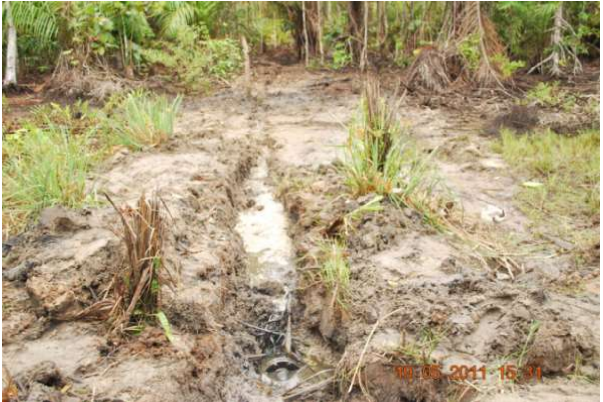
Overview: Overview of the 24" Trans Ramos pipeline at Odimodi. Picture was taken during JIV of 19 May 2011
